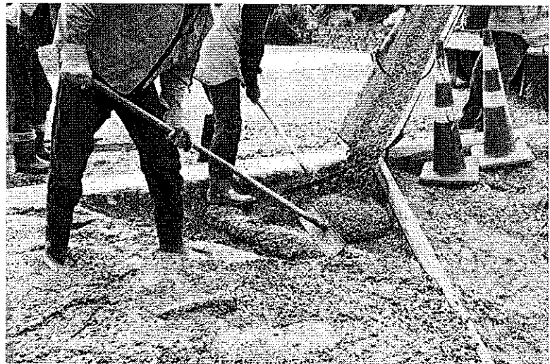
FIGURE 7. The purpose of the concrete spreader is to place the concrete as close to the finish level as possible.
